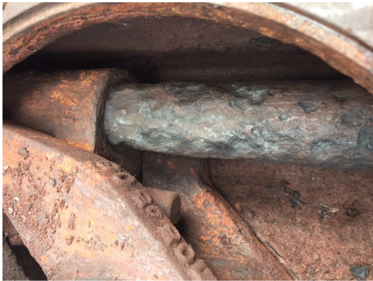
Support Rod Corrosion
